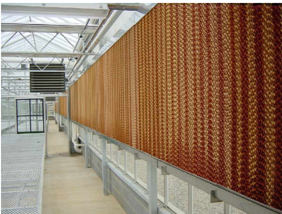
Figure 2. Evaporative cooling pads.
