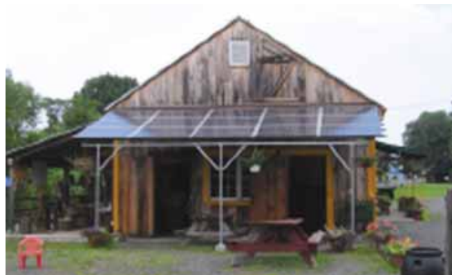
Figure 1. Photovoltaic modules were added to an existing structure to power a produce cooler within the building.
