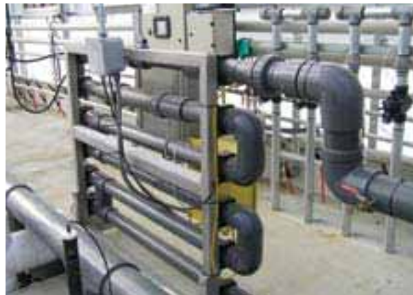
Figure 2. Organic deposits and biofilms in pipes can harbor and reintroduce pathogens.
